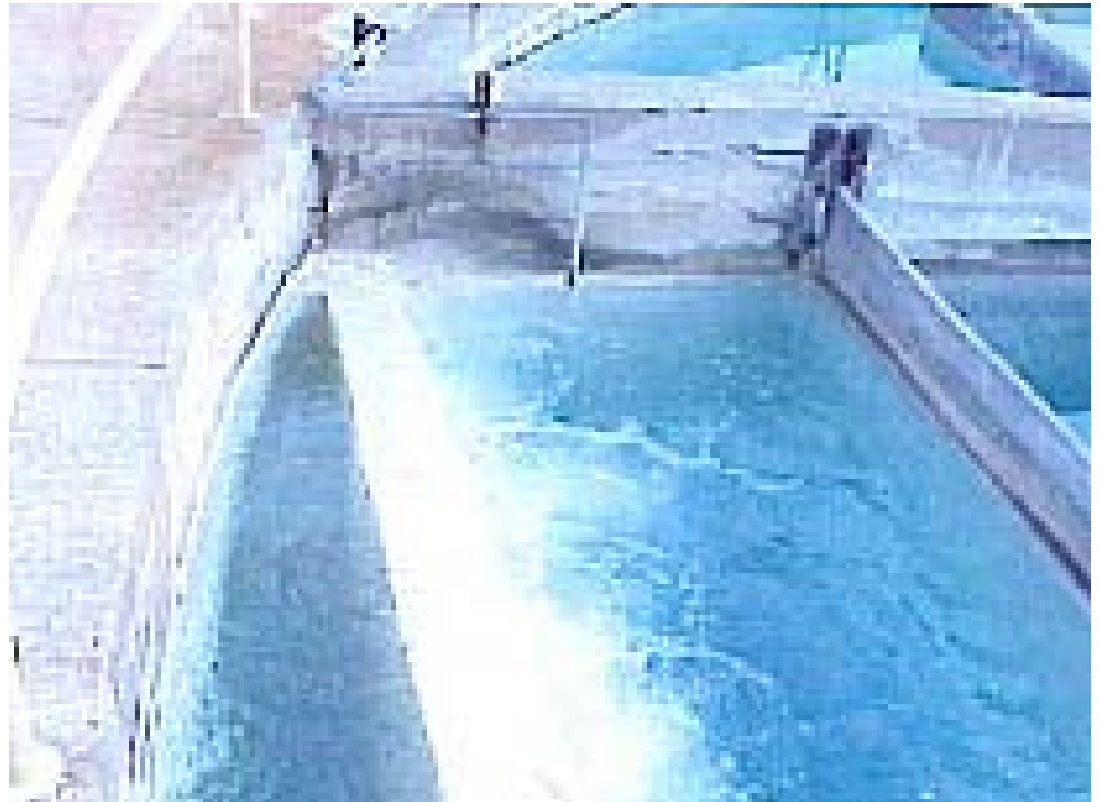
Figure 5: Re-carbonation Basins: (a) Influent to Recarbonation Basin and CO 2 Injection, (b) Main Reaction Basin.
