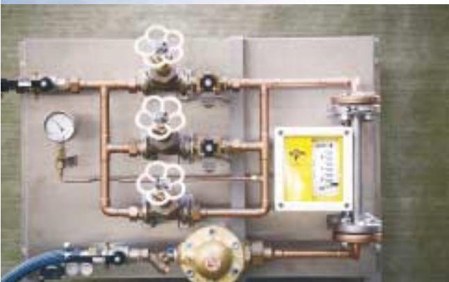
Oxygen measurement and control panel
