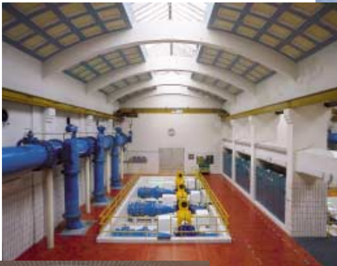
Pumping station in a waterworks
