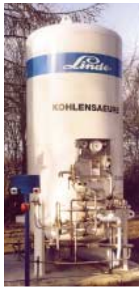
Carbon dioxide tank
