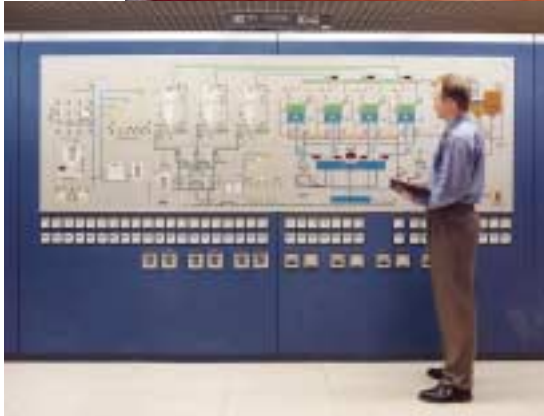
Control room in a waterworks
