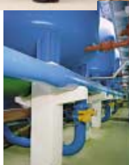
Pressure filter in a waterworks
