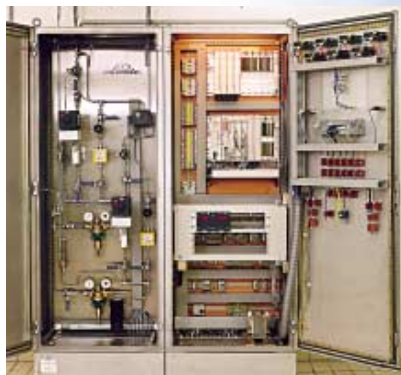
Control cabinet for the dosage of carbon dioxide
