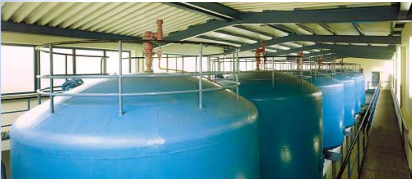
Pressure filter for the removal of iron and manganese
