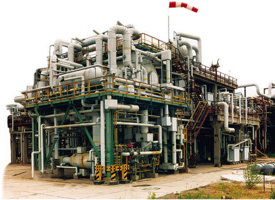
Fig. 1: Claus plant at Leuna
