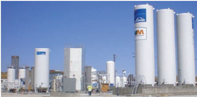
13,000 gallon per day LNG plant in Altamont, California (start up in 2009)
